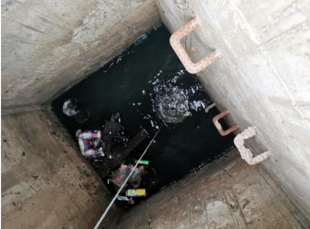
Blackish and smelly water at inlet sump
